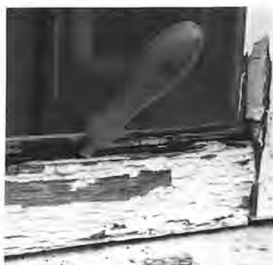
A SHARP INSTRUMENT IS ESSENTIAL IN INVESTIGATING THE EXTENT OF DECAY IN A WINDOW. IN THIS CASE, DECAY HAS FOLLOWED THE BREAKDOWN OF PAINT AND GLAZING PUTTY ALLOWING THE INGRESS OF MOISTURE.
