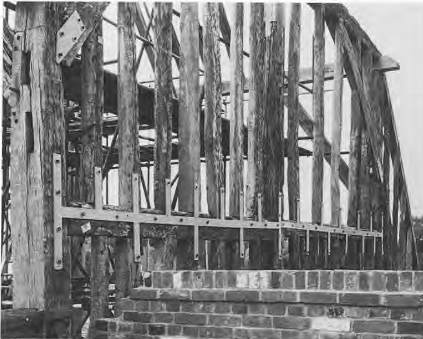
East end of Coggeshall Barn. This frame had collapsed. In its repair the use of steel strapping allowed much timber to be saved. The strap shown above is purpose-made and is covered by the external weatherboarding.
