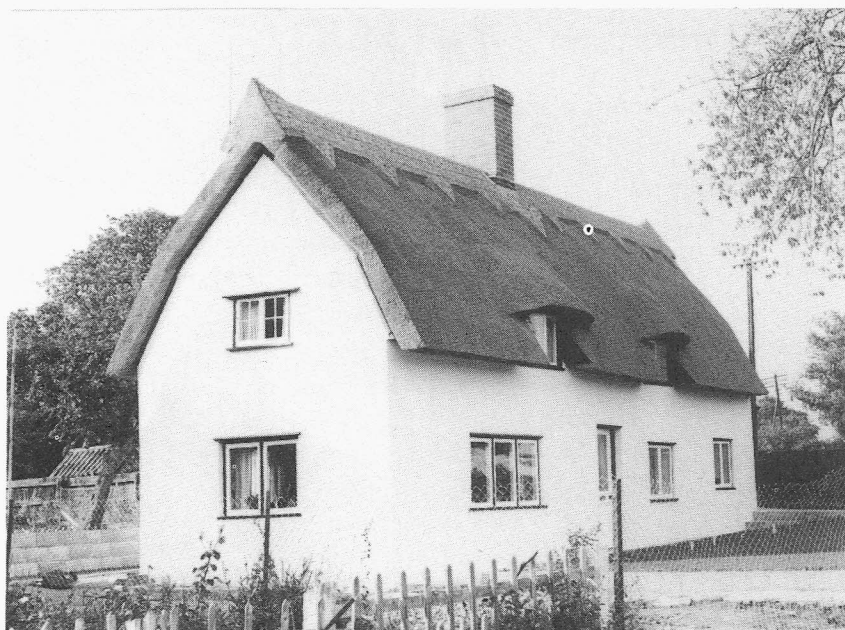
Fig. 3: Water reed thatch. The thatched mansard roof with patterned ridge is usually found in East Anglia
