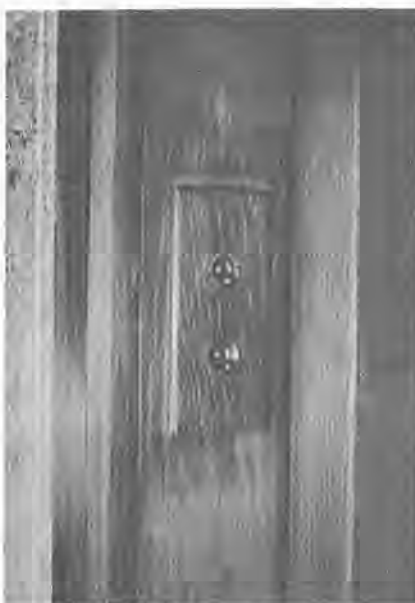
Fig. 8: Switches at Castle Drogo: retained in the rewiring.
