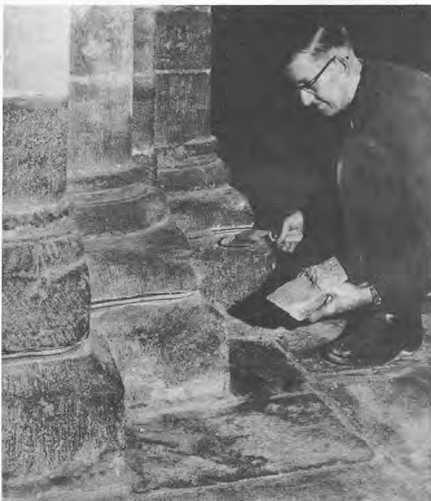
Fig. 13: A suitably wide mortar joint has been raked out to allow the MIMS cable to be run around this pier without cutting across any mouldings. Careful pointing with mortar matching the original disguises the cable run. (Photo courtesy of British Insulated Callender's Cables Ltd)
