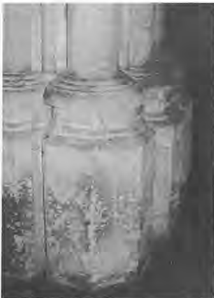
Fig. 15: Wiring at Dorchester Abbey: Cables follow the line of the mouldings, but perhaps there was an alternative route. Damp has eroded the copper clips — they should be made of stainless steel, or be PVC coated.
