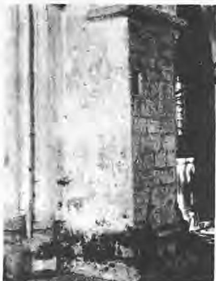
A band of dampness and discolouration usually 300 to 900 mm above ground level suggests an absent or defective damp-proof course
