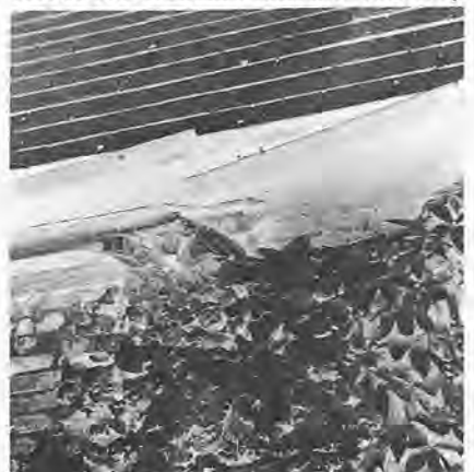
Destructive effects of unmaintained guttering
