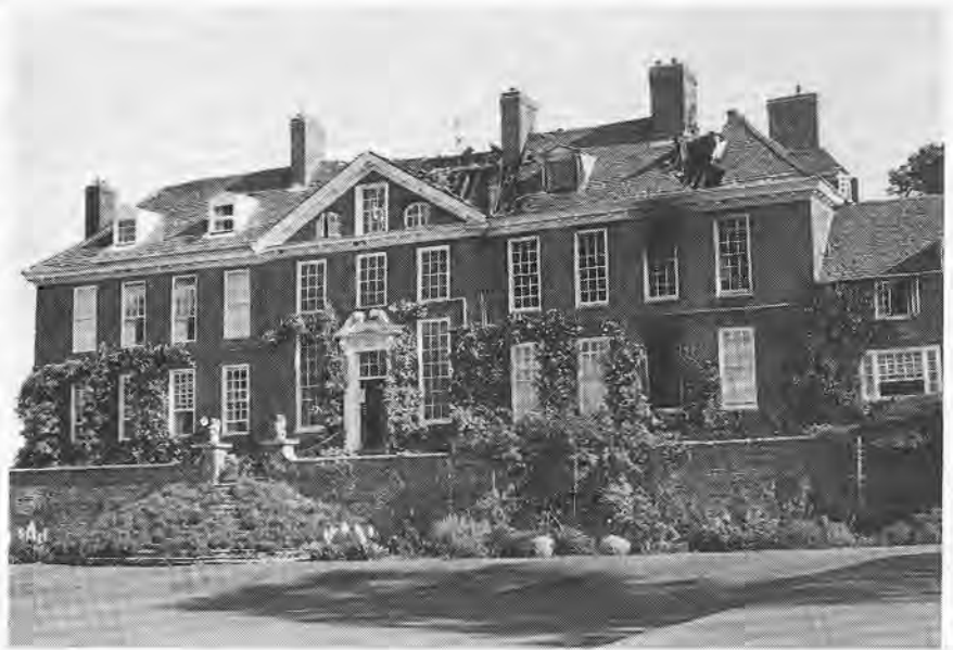
Lowesby Hall, Leicestershire: Fire damage resulting from a workman stripping paint with a blow lamp
