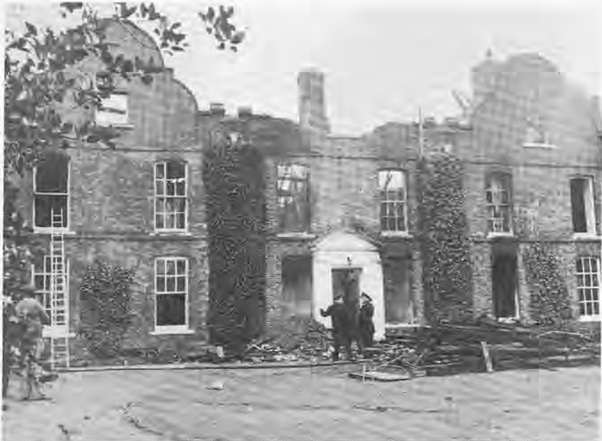
Fingringhoe Hall, Essex: The front elevation showing the destructive results of fire, but sufficient remains to rebuild
