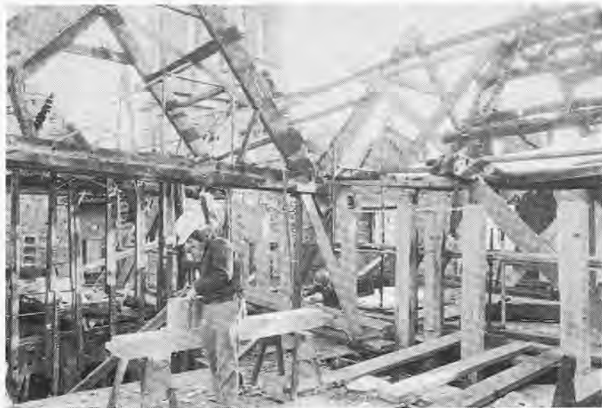
Hay Castle, Herefordshire: Workmen repairing the roof after the Castle was gutted by fire
