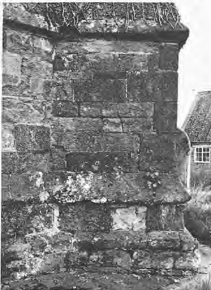
Wall in need of careful repointing
