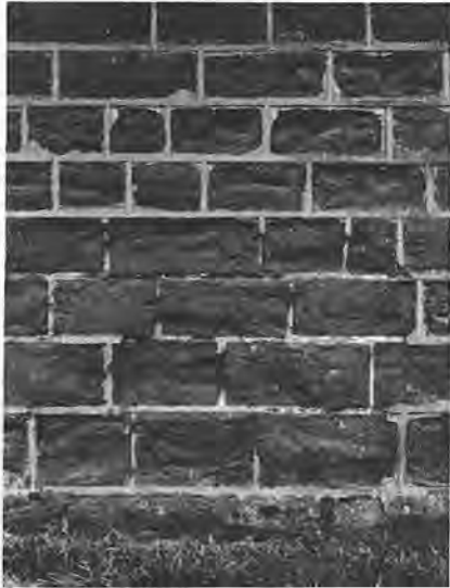
Erosion caused by impervious cement mortar limiting evaporation to the face of the stones
