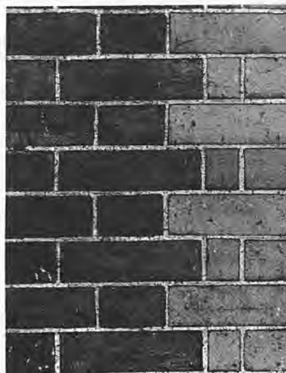
Pointing done at the time of original construction showing flush pointing in high quality brickwork with narrow joints and good arrises
