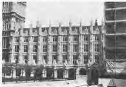
fig. 2: New Palace Yard, Palace of Westminster, showing Anston, Clipsham and Portland stone cleaned by intermittent washing and small "suction gun" air abrasive tools. This is a typical successful combination of two methods.
