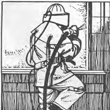
fig. 5: Acid clean general: the Craigleith sandstone is being cleaned with solutions of hydrofluoric acid and some limited abrasive blasting in support.
