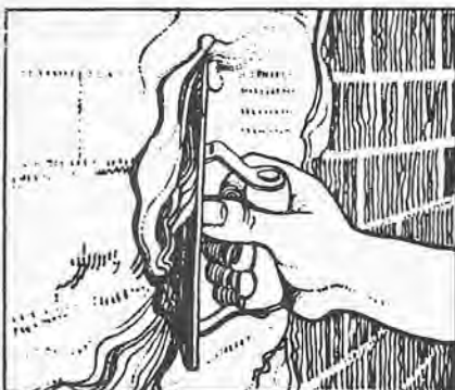
fig. 9: Application of clay poultice: the wet clay has good adhesive properties, and may be thrown onto the wall, before spreading evenly with a float to an average 15-20 mm thickness.
