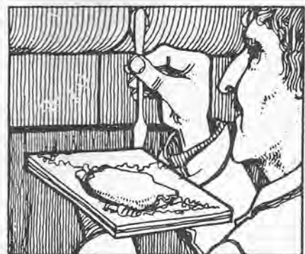
fig. 11: Pointing up fine joints and cracks with non-shrink mortar before cleaning: preparation of this kind is essential and should precede the start of any cleaning operation.
