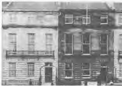
fig. 6: Craigleith sandstone terrace houses in Edinburgh show the typical cleaning effect achieved by the use of dilute hydrofluoric acid; the dark staining in saturation zones is an unfortunate effect of weathering which cannot be removed and must be anticipated on some light coloured sandstones.
