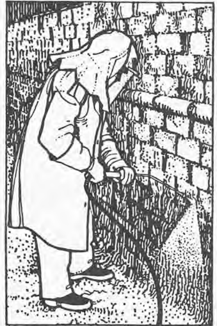
fig. 8: Chemical cleaning using caustic alkali: the operative, properly clad for chemical handling, is using a high pressure low volume water lance to wash off the alkali.
