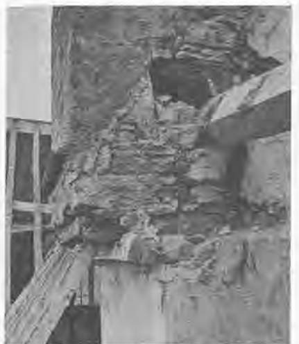
Above: General view of the central chimney stack at Kelmscott Manor. Below: Detail of the defective supporting timbers revealed on opening up (see Fig 6).
