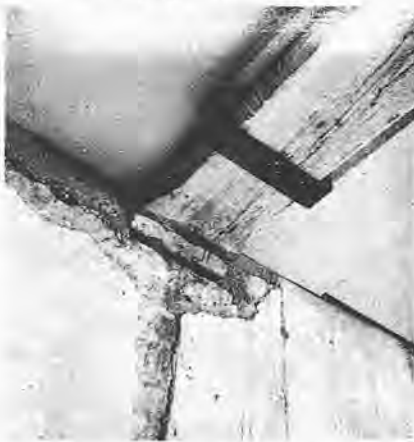
Fig. 13: A cradle of steel plates was used to support beams at Knole, in Kent
