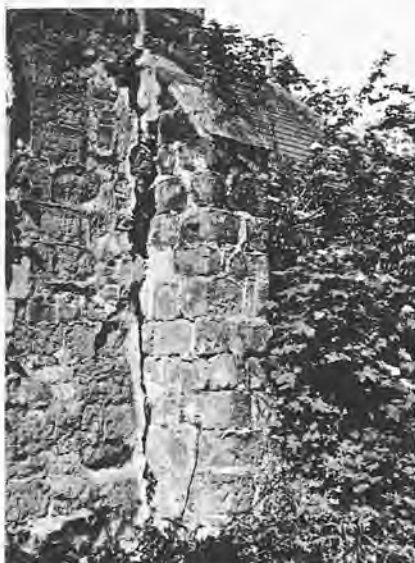
fig 4: Buttress failure at All Saint's church, Malby le Marsh, Lincolnshire
