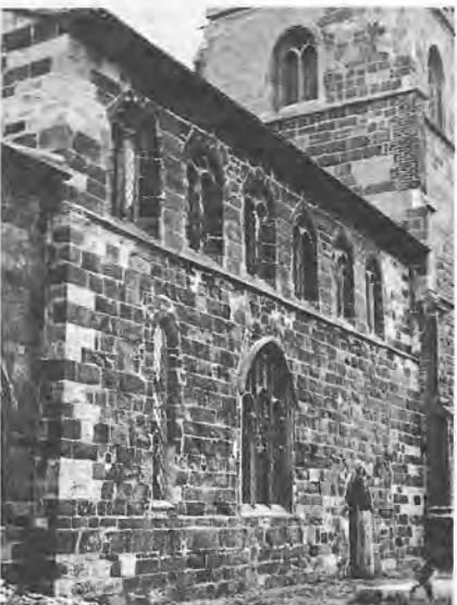
figs 16, 17 and 18: The progress of the work of pulling back the north wall of Orby church
