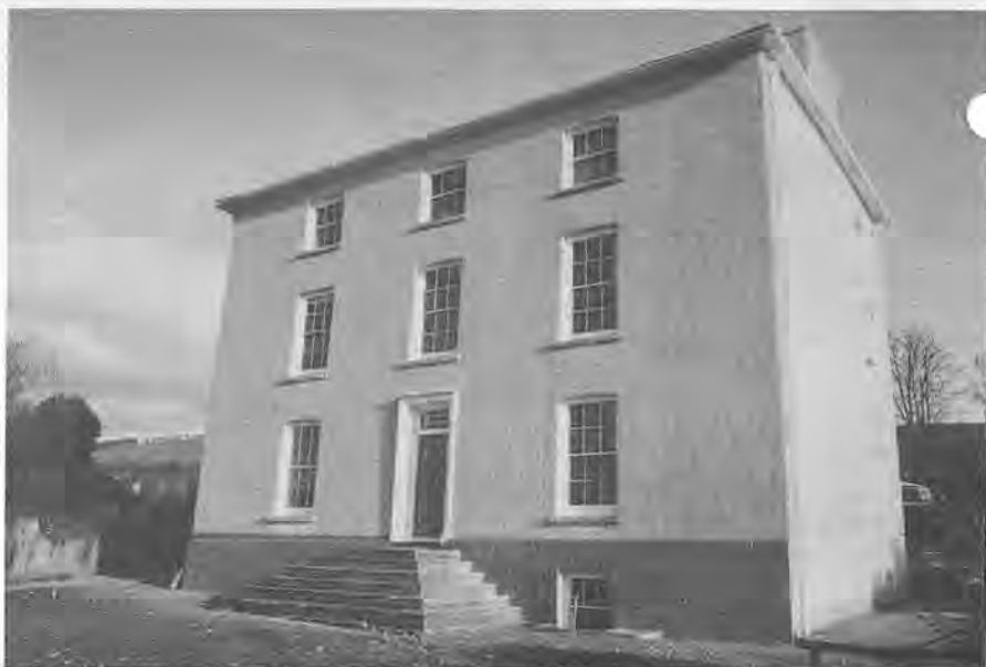
Bryn-y-mor House, Cardiganshire: the use of cement-based mortar and paint increased the quantity of driving rain passing, by capillary action, through the exposed slate walls of this house. Following removal of these earlier 'repairs', lime-based rough-cast and limewash have been applied with successful results.
