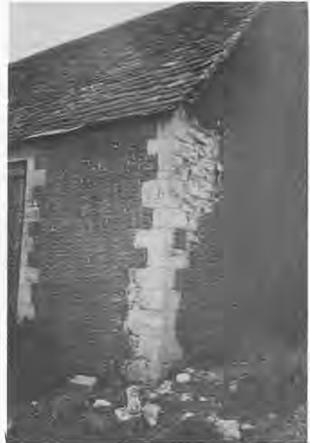
Frost action on moisture trapped behind cement-rich rough-cast has led to the disintegration of rubblework and dressed quoins with the rough-cast peeling off in large sheets.
