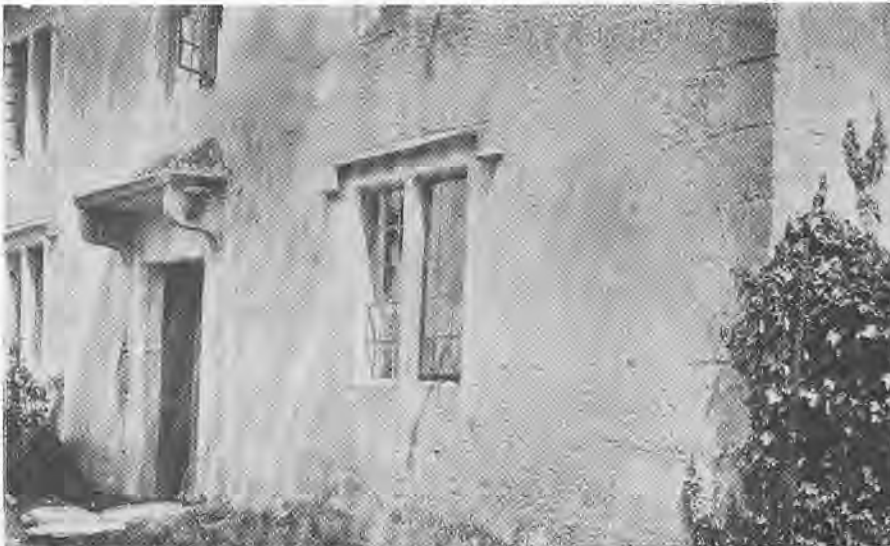
A good rough-cast surface dying out onto the quoins of a rubble-built wall from a cottage at Castle Combe.
