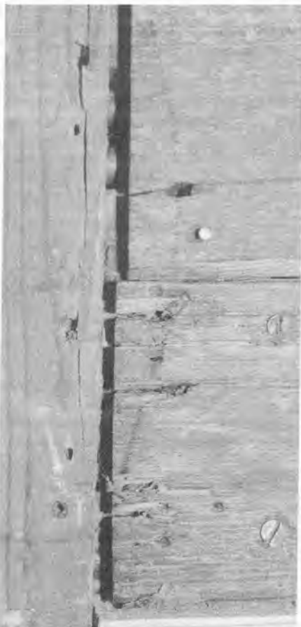
Board damaged by careless lifting and relaying during installation of central heating and wiring runs (pipes and wires just visible in gap between boards).
