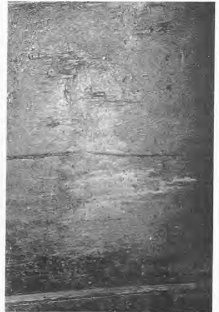
Damage to board caused by a castor. This can be particularly serious when the castor is positioned over the edge of a board.
