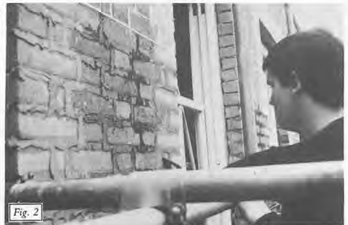
Base mortar nearing completion. Note different tones for reveal and main brickwork. Surplus mortar has yet to be cleaned off before grooving takes place.
