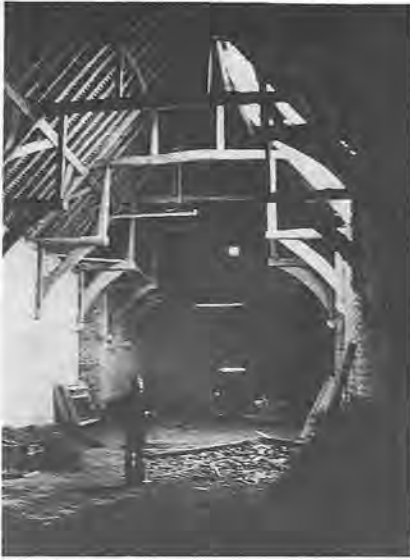
Rot at junction of purlin and principal rafter led to collapse of one whole bay of the roof.
