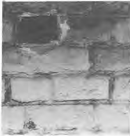
Multiple layers of oil-bound paintwork has prevented evaporation of moisture within the wall. Limewash would have allowed the wall to "breathe".
