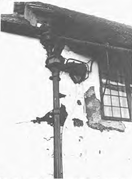
Frequently overflowing hopperhead and gutter have saturated the wall behind an impervious paint layer. Decay of the walling immediately behind the paint film has resulted in flaking.
