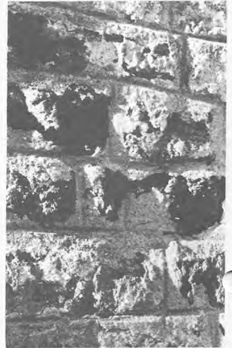
Dense cement pointing splurged over the face of the stonework inhibits the evaporation of water from the wall and leads to rapid decay of the stone.
