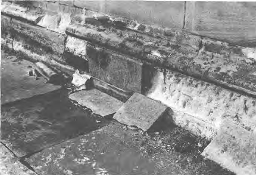
Salt crystallisation behind the strong cement patches on this plinth has led both to these being forced off and to further disintegration of the stonework.
