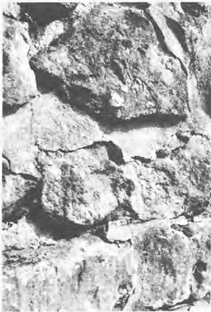
Strong cement pointing being forced off the wall by crystallisation of salts behind. Increased levels of dampness within the wall have caused decay of the earth-lime mortar, leading to compaction of the wall—also forcing off the dense pointing.
