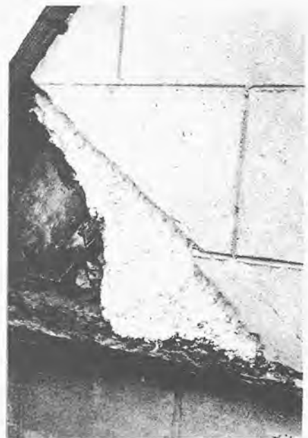
Cement render has been applied over a lime roughcast on this timber-framed building. The cement is being carefully removed in small pieces by forming hairline cracks with a lump hammer.
