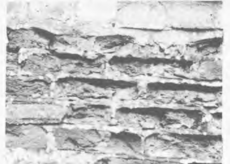
Strong cement-based mortar survives while the wall it was used to point-up decays. This could have been avoided by the use of a lime-based mortar, weaker than the brickwork.
