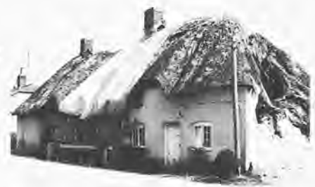
Water penetration at the top of the cob walls has resulted in their decay. The cement render applied externally prevented the walls from drying out and led to the suddenness of the collapse.
