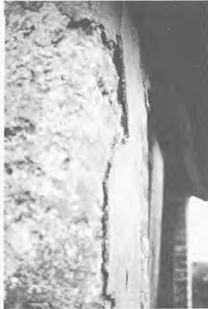
Strong cement render on a cob wall. The render is being forced off the wall and is taking the surface of the cob with it. The cob behind this is decaying.
