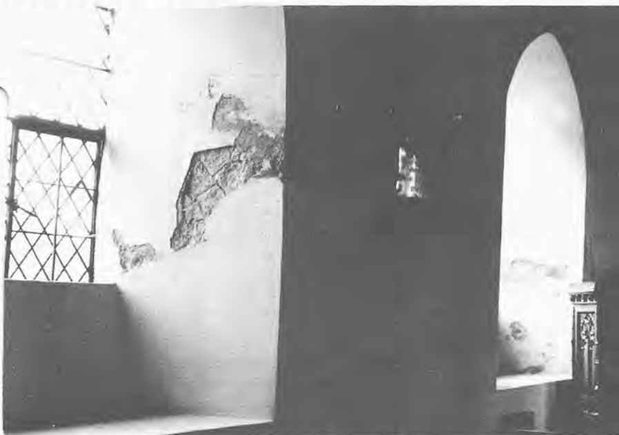
Strong cement-based render has been used to replace plaster affected by damp on the lower part of these massive walls. As a result the damp has risen higher in the wall and has now affected old plaster that had remained sound.
