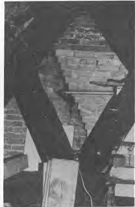
The heavy smoke blackening and soot encrustation is evidence of an early date for this building. A hearth in a hall open from ground to roof without a chimney would have produced this effect. The chimney in the background is a later insertion.
