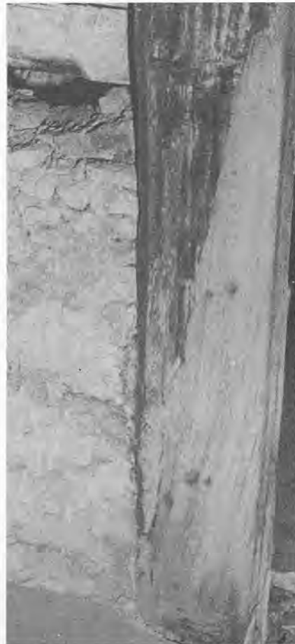
A once fine main post resembles a tree trunk after all frassy timber has been cut away.
