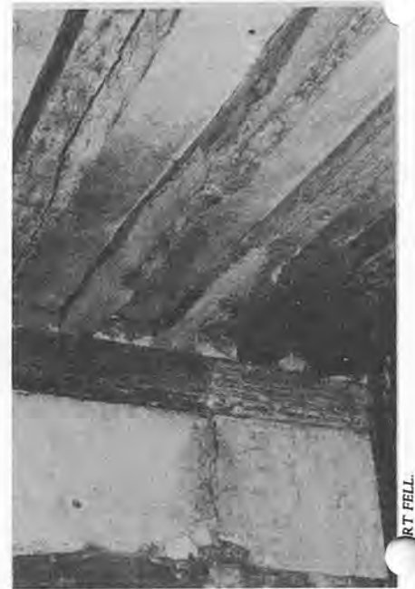
Defrassed fine square section medieval floor joists now resemble poor quality 'pole' construction.
