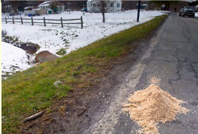
Exhibit 3-11: Road salt can contaminate surface and ground water.
